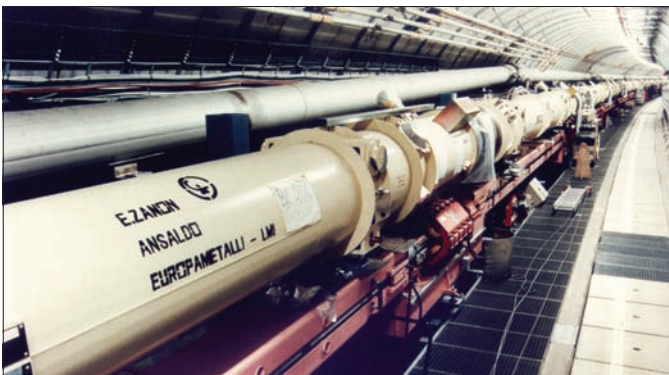
A view inside the 6.3 km tunnel of HERA shows the superconducting magnets – used to guide the proton beam – installed above the normally conducting magnets of the electron ring. (Courtesy DESY.)
